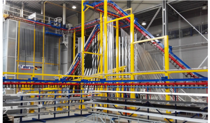
Vertical and horizontal powder-coating shops
